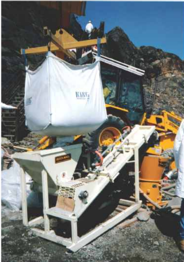
Figure 3: Bagged pre-mixed dry shotcrete components being delivered into a hopper feeding a screw conveyor, fitted with a pre-dampener, which discharges into the hopper of a shotcrete machine
