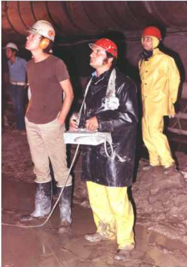
Figure 11: Shotcrete operator using a remotely controlled unit to apply shotcrete to a rock face in a large civil engineering excavation.
